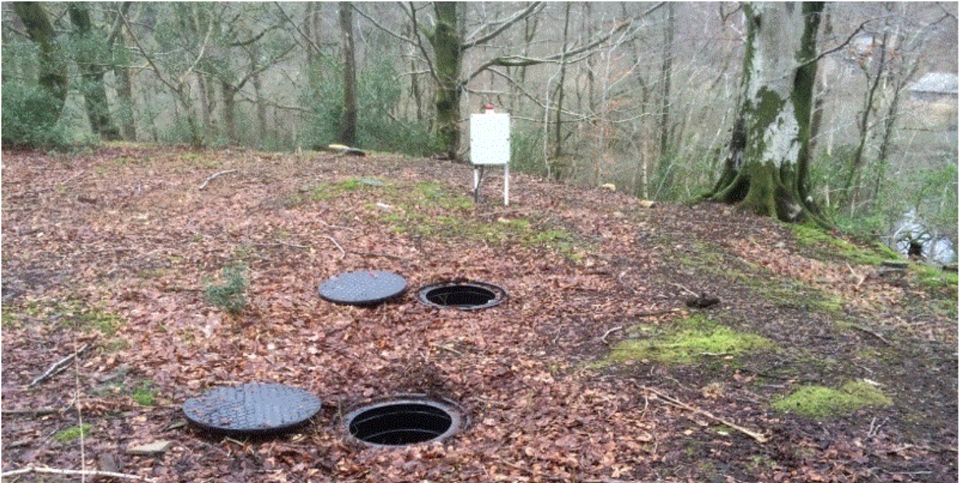
Figure 1. Private domestic sewerage system covers (photo kindly provided by Hutchinson Environmental Solutions).
